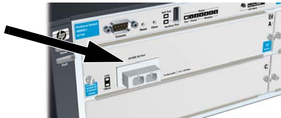
Figure 8. X2 transceiver fully installed
