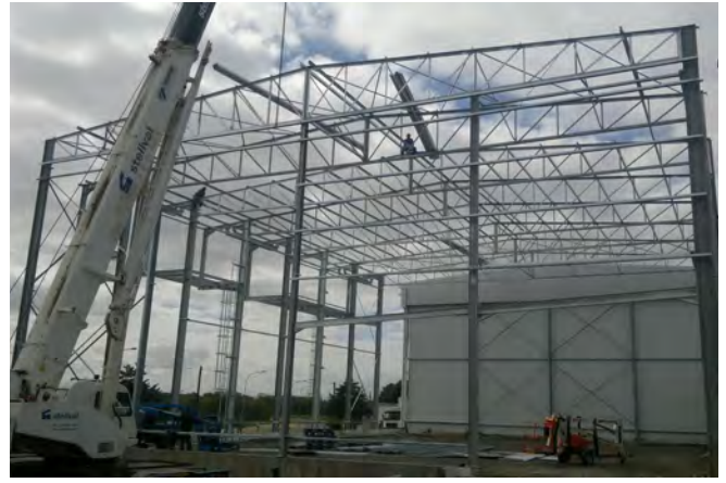
Leading Edge Engineering specialises in the engineering, manufacturing and fabricating of all types of steel products and structures and also does project management
