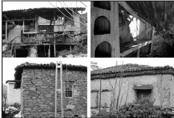
Figure 14. Examples of Structural Problems in Unused Houses.
