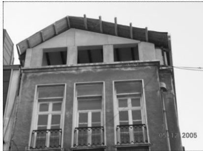
Figure 4. Illegal Floor Additions to a Historic Building (Karabetça, 2005).
