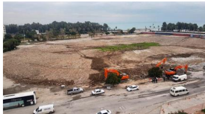
Figure 2. Mersin Tevfik Sırrı Gür Stadium after the Destruction.
