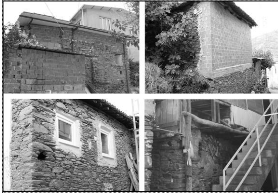
Figure 13. Examples of Repairs Made with Inappropriate Materials (Repairs on the Roof, Wall, Window Profile and Staircase).
