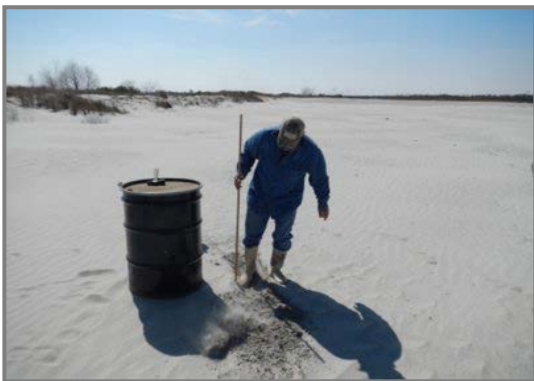
Electrician installing grounding wire for MPPEH Storage Area on ICW Dredge Spoil Island
