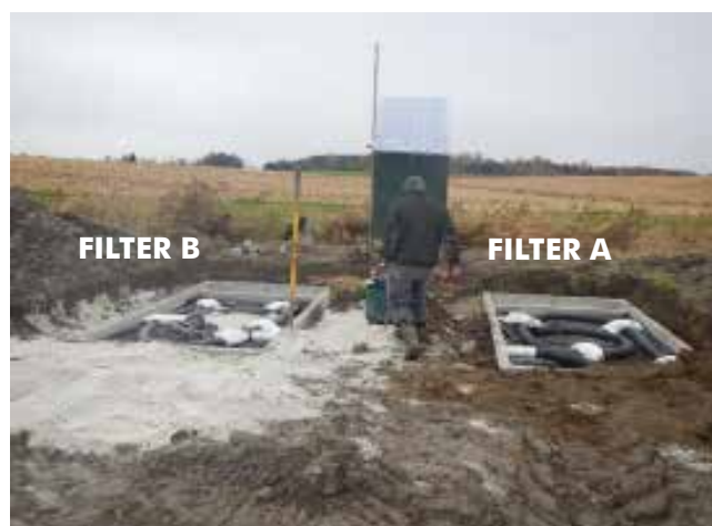
Phosphorus filters filled with media, prior to placing on lids. Filter B (left) was comprised of limestone “bedding sand” and Filter A (right) contained drinking water treatment residuals.
