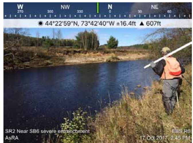
Assessing a severely eroded and actively eroding bank that blocks access to a key floodplain in the Town of Jay on the East Branch of the Ausable River.
