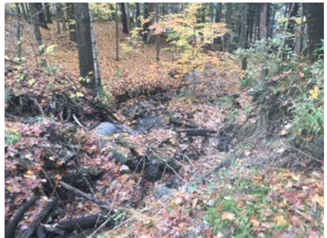
Failed culvert at site, one of several projects to be addressed
