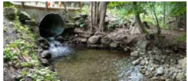
This photo shows the current culvert in its current state taken in summer of 2017.
