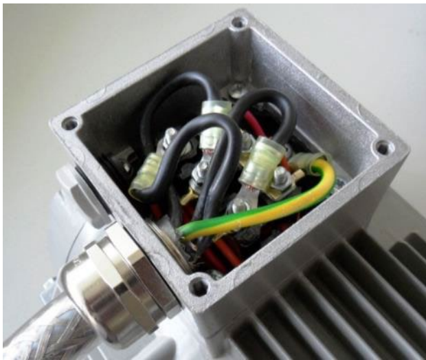
Fig. 22: Wiring on the motor connection box
