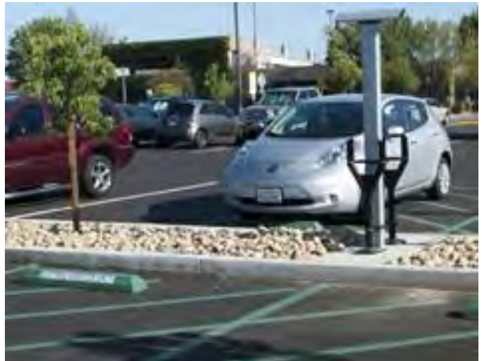
Electric charging station in Bakersfield
