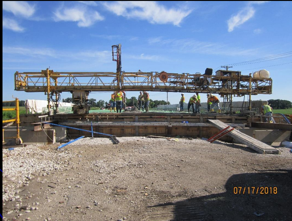
Bridge crews set reinforcement bars, pump concrete to the deck and use a paving machine to strike off the deck on the new bridge for the West County Line Rd over Union Ditch #3 Bridge Replacement project
