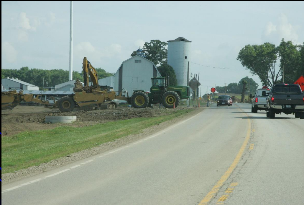
Flaggers control traffic as scrapers and quarry trucks move dirt from west to east, while utility relocation and sewer installation continues on the project on LMP Section B-2
