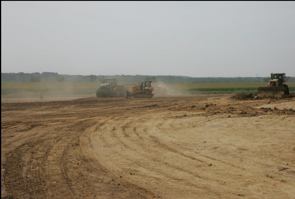
Earthmoving operations at the Raging Buffalo site continue on the LMP Section B-2 project
