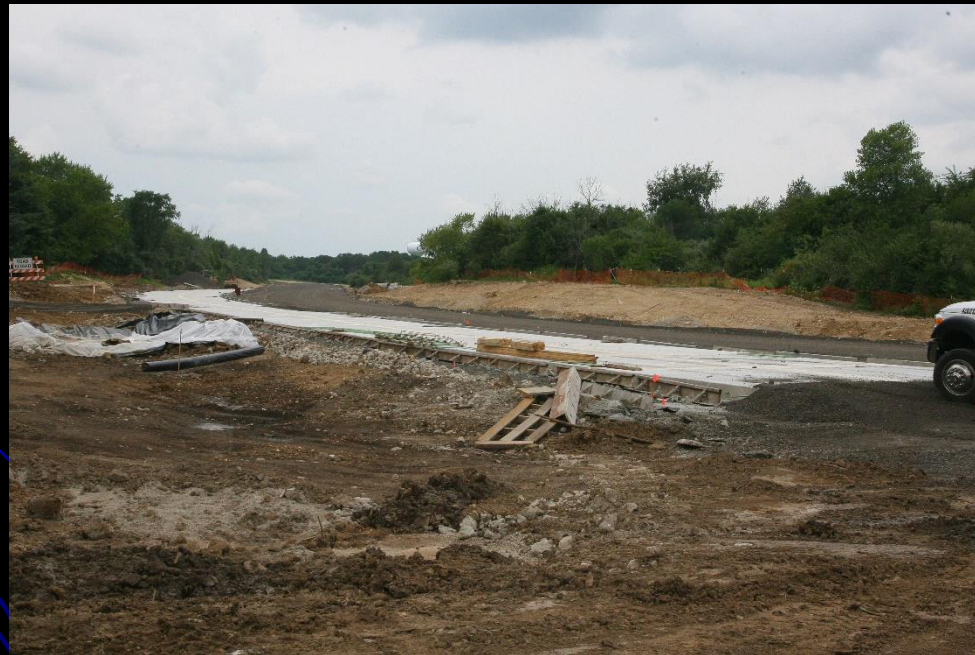
Crews set forms and pour a small section of the new pavement for new Longmeadow Parkway on the LMP Section D - IL 25 to IL 62 project
