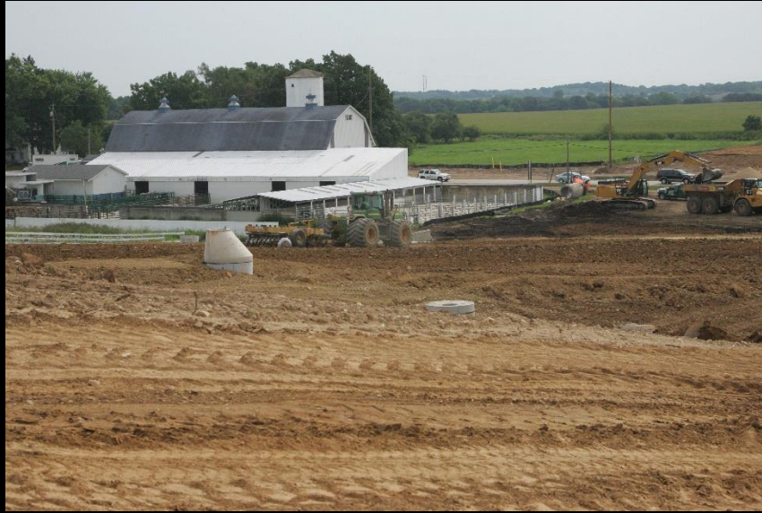
Earth moving and processing is in full swing on the LMP Section B-2 - White Chapel to IL 31 project
