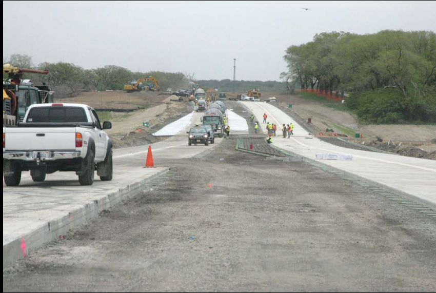
Crews pour turn lanes for the new concrete pavement east of White Chapel on the LMP Section B-2 - White Chapel to IL 31 project
