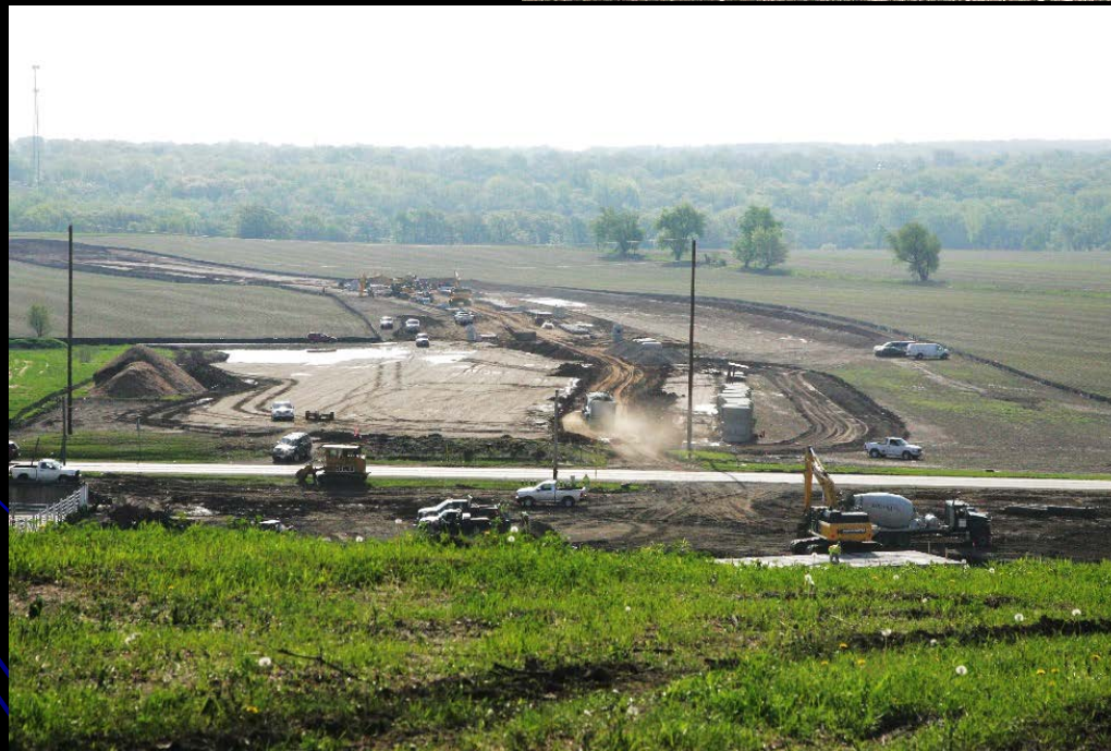
Crews build box culverts and install new storm sewer lines for the new roadway east and west of IL Route 31 on LMP Section B-2
