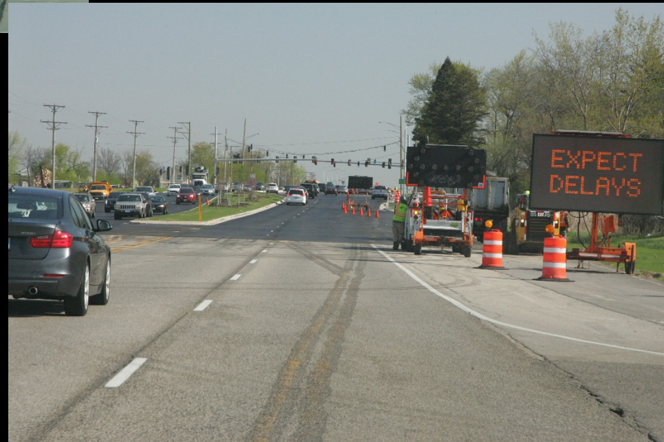
Asphalt surface is placed on Randall Road as the contractor completes work for the LMP Section A-2/B-1- Randall to Karen Drive project
