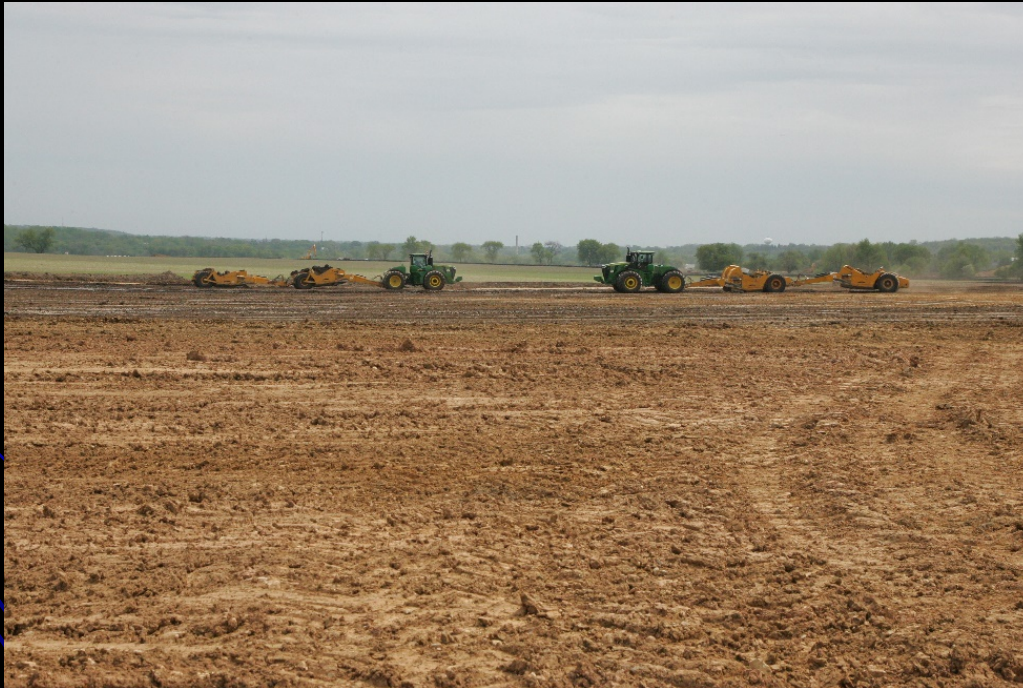
Earth moving operations at Raging Buffalo are in full swing as crews prep the subgrade for embankment on LMP Section B-2
