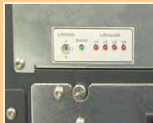
Fan failure display/ four speed levels
