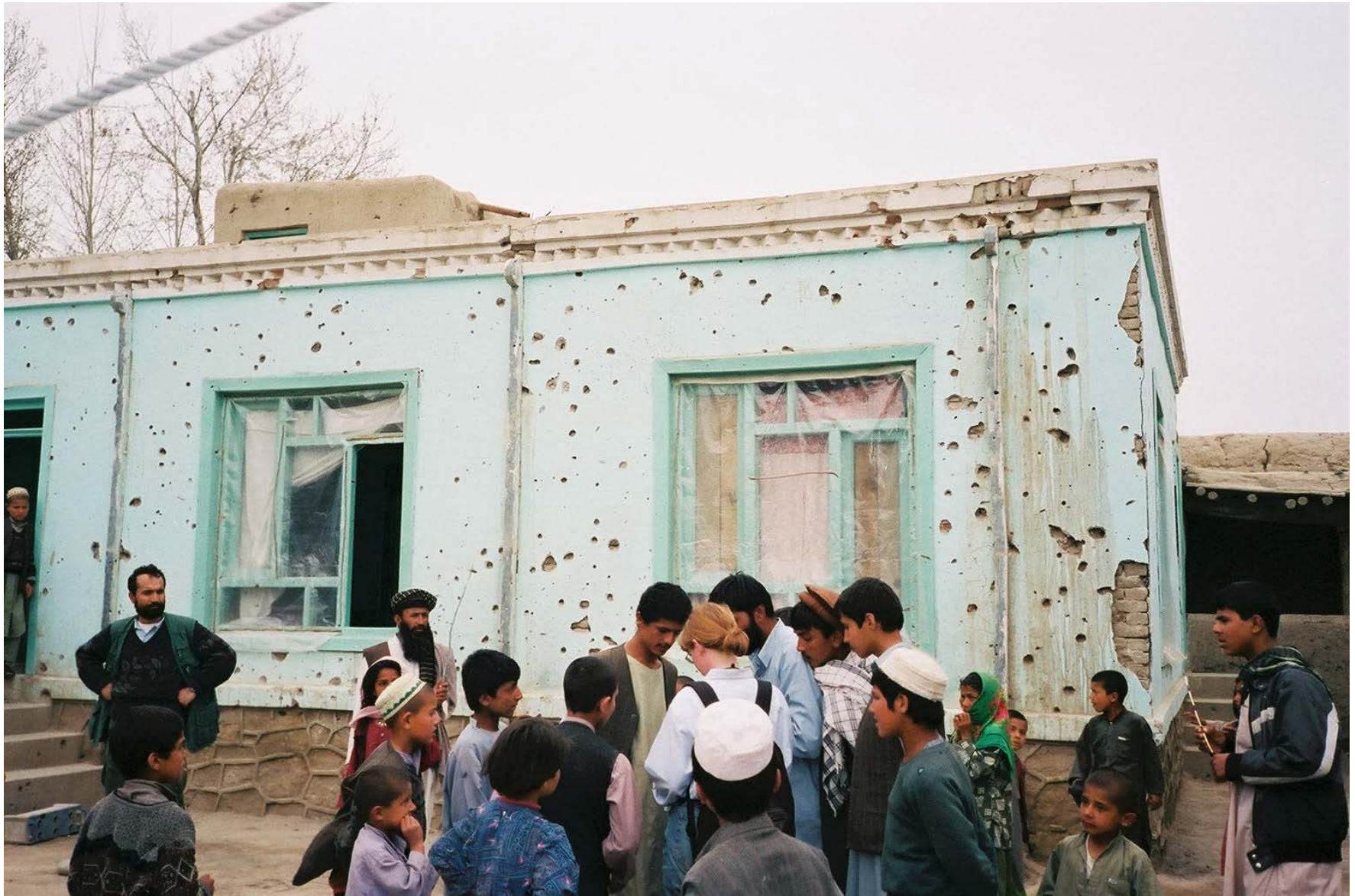
Cluster bomblets left pockmarks on this home in Ainger. Some pieces of shrapnel penetrated the house and made holes in a bedspread. © Reuben E. Brigety, II / Human Rights Watch, 2002.
