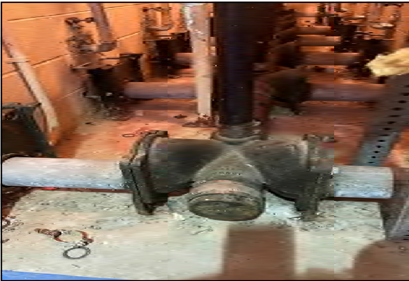
5) View of assumed asbestos containing pipe connectors located in the utility closets.
