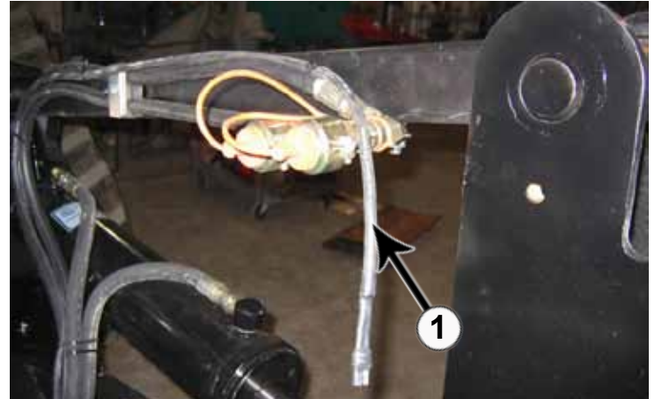
29. Guide the extension cord from the wire harness to the front of the tractor. Run the wire along the left side of the lift frame (1).
