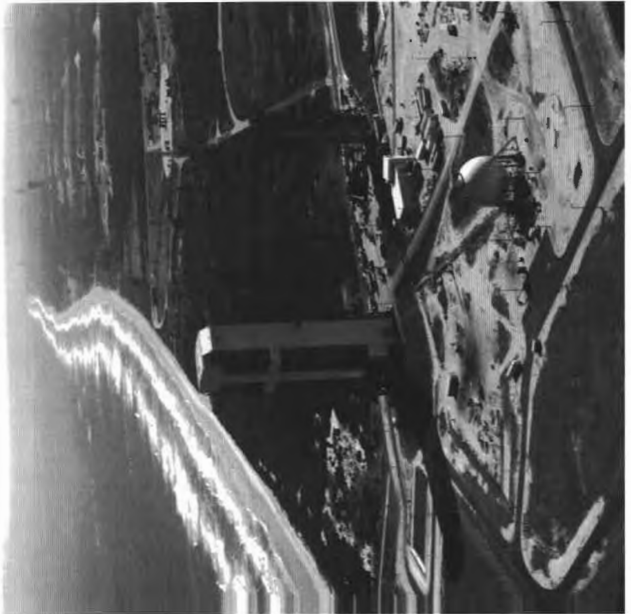
Illustration 4-4 Launch Complex 37 under construction at Cape Canaveral, February 2001, Delta IV Launch Tower at center (Boeing Company photograph)
