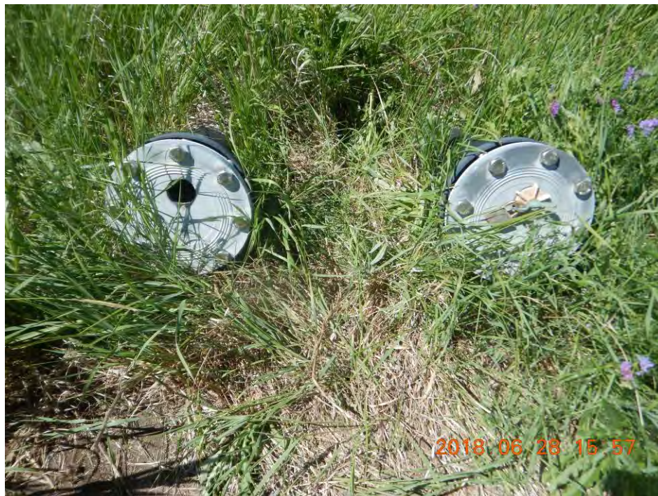
Photo 30 – Leachate Collection and Leakage Detection System (LCS and LDS) Access Pipes South Side – Missing LCS cap and lock.
