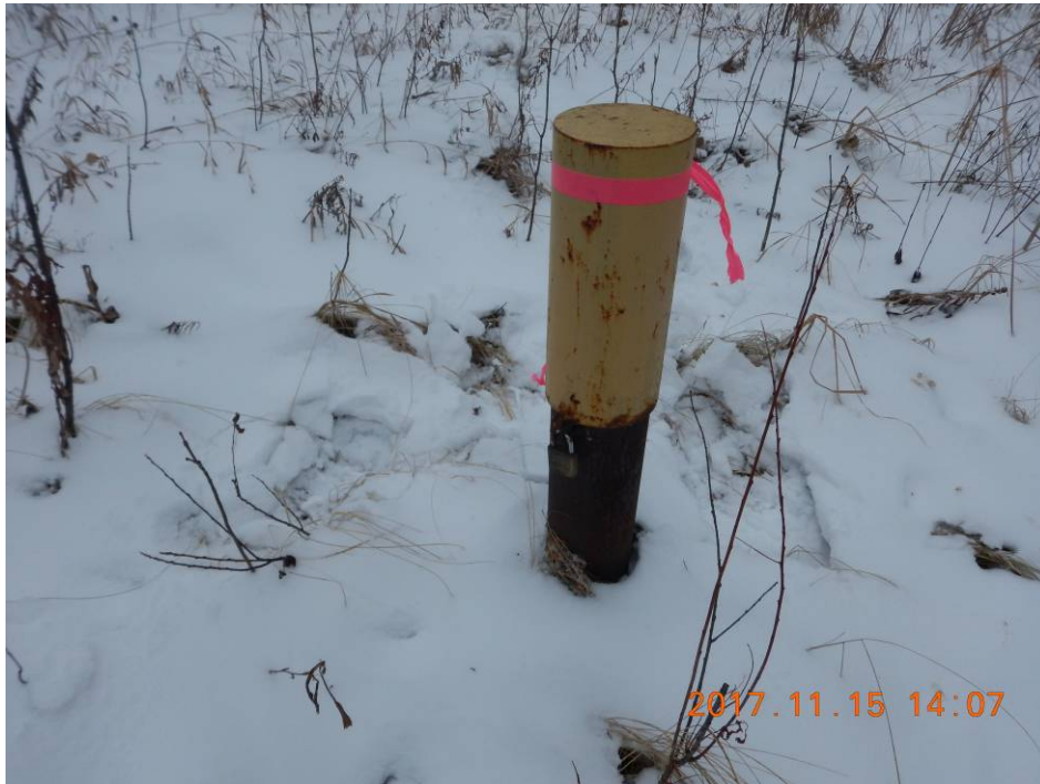
Photo 15 - Well 2000-B1 – Casing Locked
