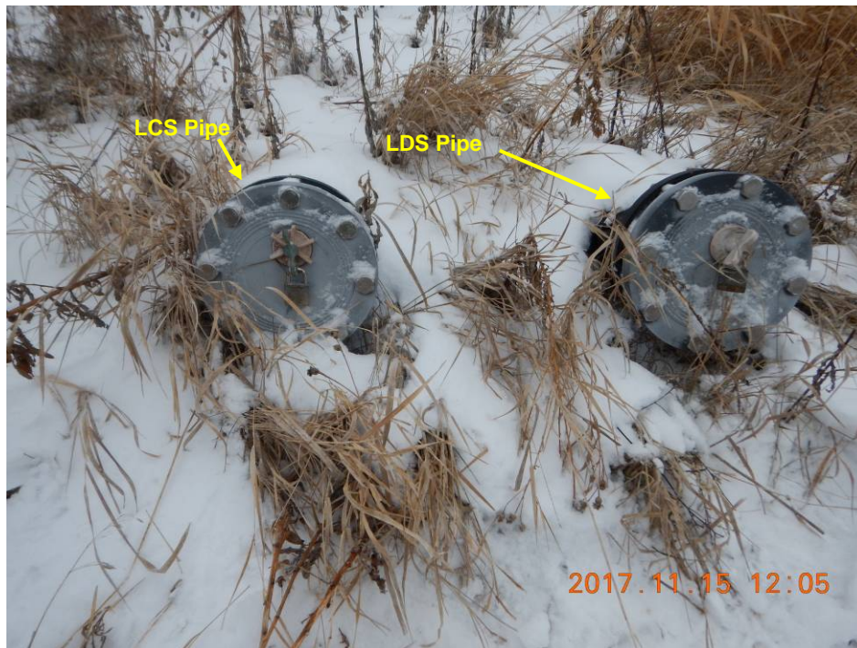
Photo 30 – Leachate Collection and Leakage Detection System (LCS and LDS) Access Pipes South Side – Locked and Secure
