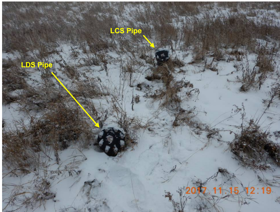
Photo 29 – Leachate Collection and Leakage Detection System (LCS and LDS) Access Pipes North Side – Locked and Secure
