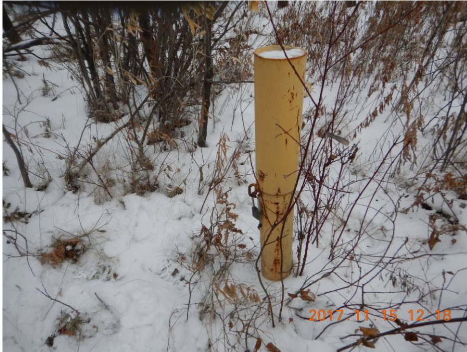
Photo 27 – Well 99-Cell-3 – Casing Locked
