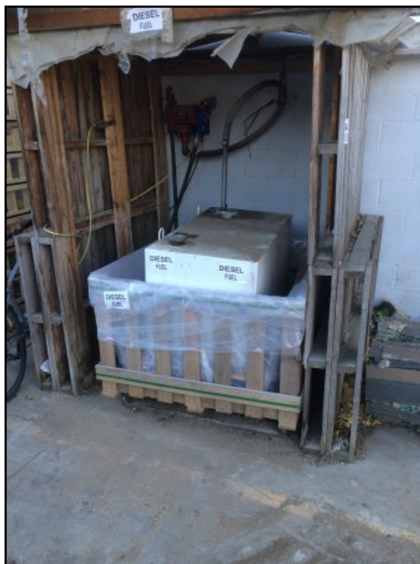
Diesel fuel storage tank with makeshift secondary containment.
