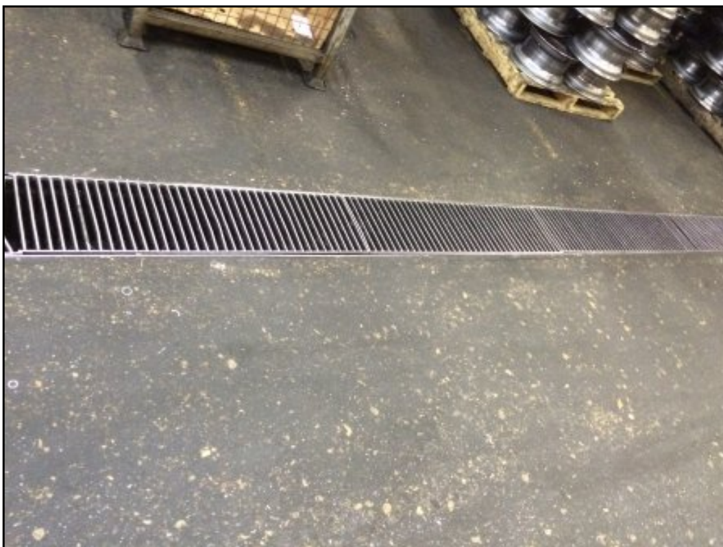
Floor drain in wheel fabrication area.
