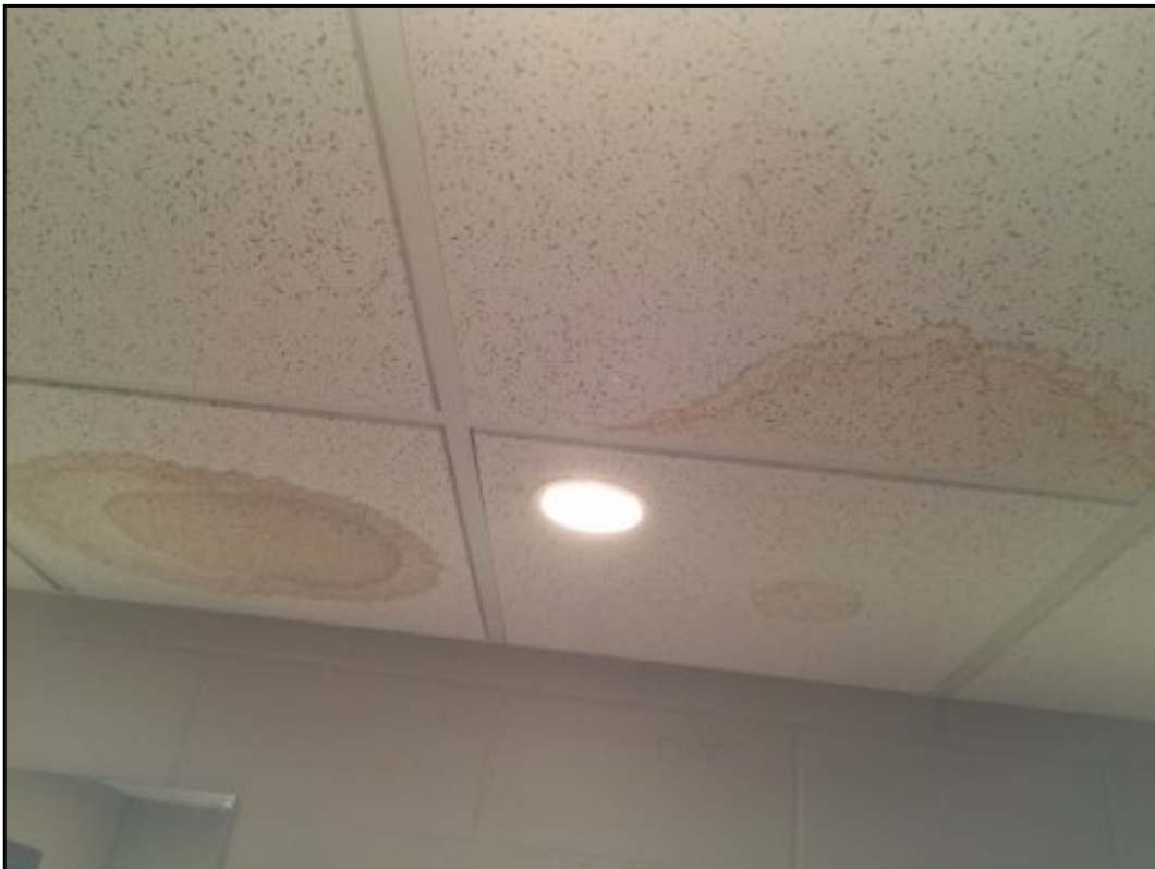
Water damage in office area.
