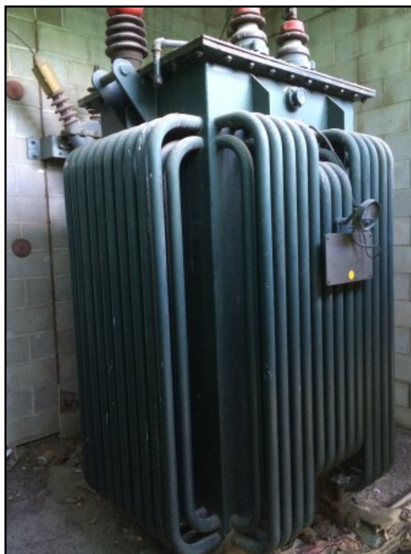
Electrical transformer with yellow sticker indicating low PCB content.
