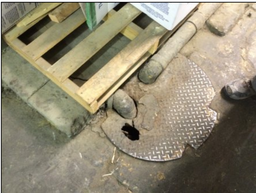
Sump pump near paint booths.
