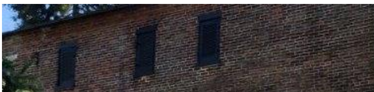
The windows on the second story of the guest house have louvered shutters.
