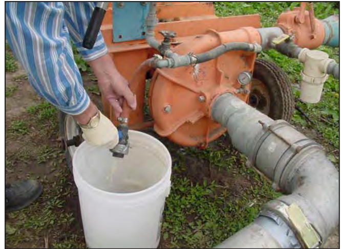
Figure 4. Liquid out of pump.
