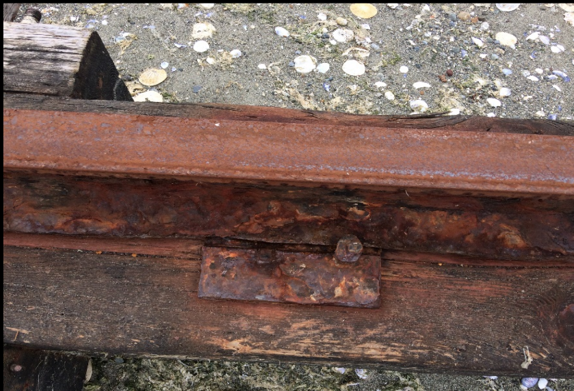
The fasteners have corroded and are failing.
