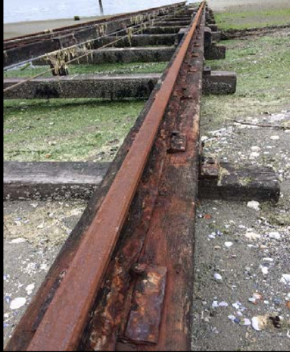
The tracks are corroded.
