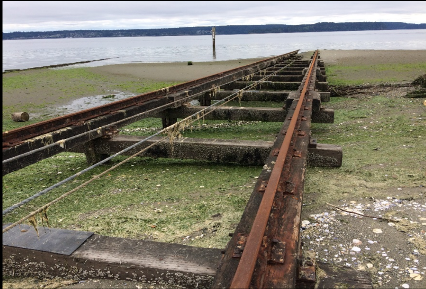
The track system which transports the ships to the dry dock.
