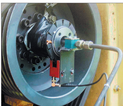
Measurement of vibration and torque through telemetry at side
