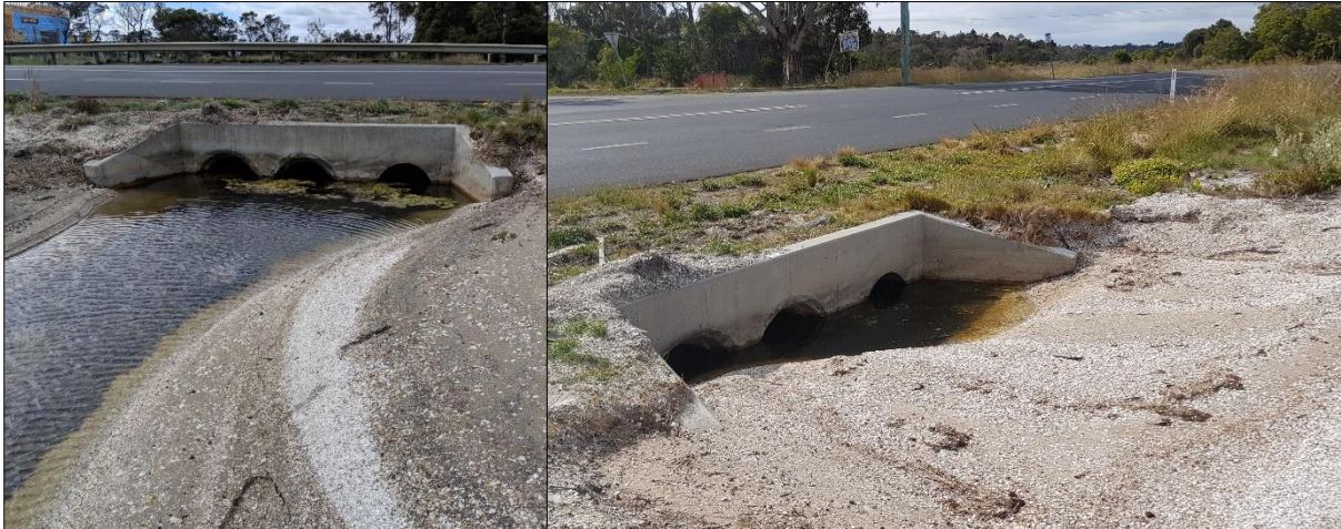
Figure 5-27. Culvert at creek line near Lauderdale Oval, between Racecourse Flat and Ralphs Bay Conservation Area. Left: previously blocked culvert on day of clean-out. Image: CCC 26 Sept 2019. Right: same culvert almost closed again. Image: DEP 10 Dec 2019.
