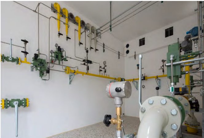
GAS MIXING CABINET OF THE GAS FEED-IN STATION (SOURCE: MAINZER STADTWERKE)
