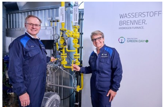
FLEXIBLE HYDROGEN BURNERS IN THE PAINT SHOP (SOURCE: BMW GROUP)
