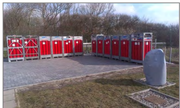
HYDROGEN SUPPLY (E.ON TECHNOLOGIES)
