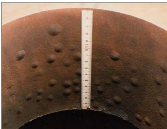
BLISTERS ON THE METAL SURFACE UNDER HIGH T EMPERATURE HYDROGEN ATTACK (KAWANO, K 2004)
