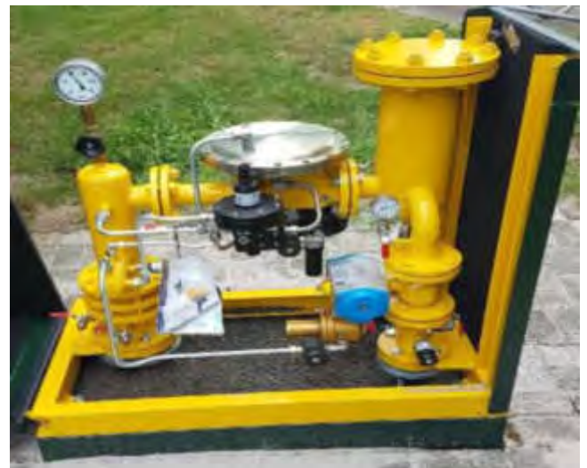
GAS PRESSURE REGULATING STATION (DISTRICT STATION) (SOURCE: KIWA REPORT)
