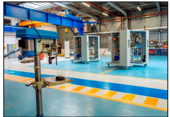
AREVA H 2 GEN PRODUCTION FACILITIES (AREVA H 2 GEN)
