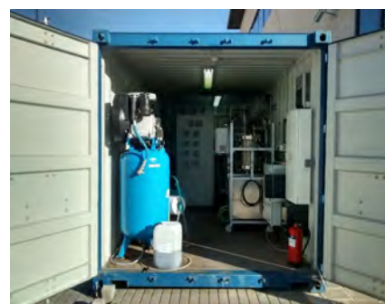
EQUIPMENT INSIDE THE CONTAINER (RENOVAGAS)
