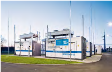
PTG FALKENHAGEN (UNIPER ENERGY STORAGE GMBH)
