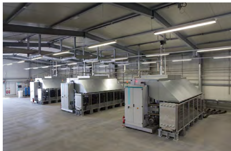
BUILDING WITH THREE ELECTROLYSERS (SOURCE: MAINZER STADTWERKE)
