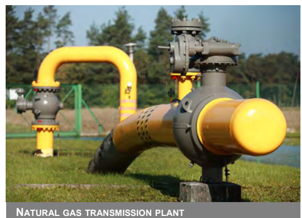
NATURAL GAS TRANSMISSION PLANT
