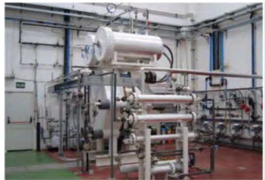
RIGHT: TEST BENCH ELECTROLYSER AT FHA FACILITIES. (ELYGRID)
