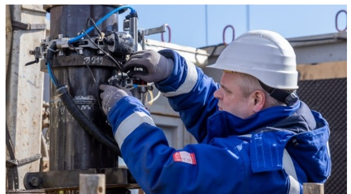
QUALITY TESTS OF THE WELD SEAMS BETWEEN THE STEEL PIPES (SOURCE: ANDREAS PRINZ)
