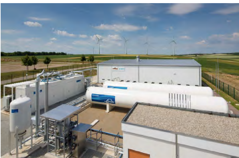
ENERGIEPARK MAINZ WITH COMPRESSOR, GAS CYLINDERS, FEED-IN STATION, ELECTROLYSER BUILDING (SOURCE: MAINZER STADTWERKE)
