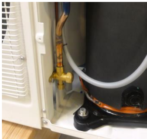
Figure 23: Liquid line service port
