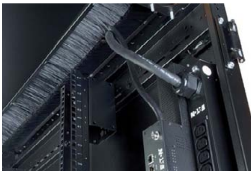
RP Series rack with 2 installed Eaton ePDUs
