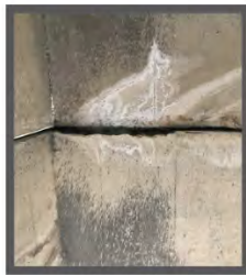
SEPARATION IN CULVERT CEILING
