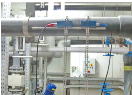
QStar's Thermal Energy Metering
