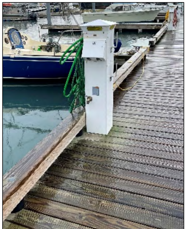
Figure 2.11: Typical combined power and water pedestal (J Float).
