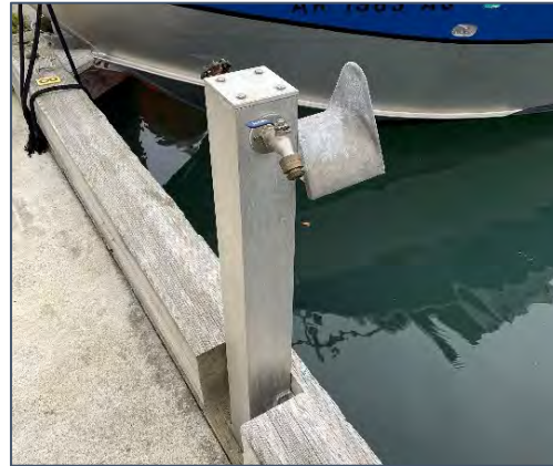
Figure 2.42: water hose bib and hose stand.
