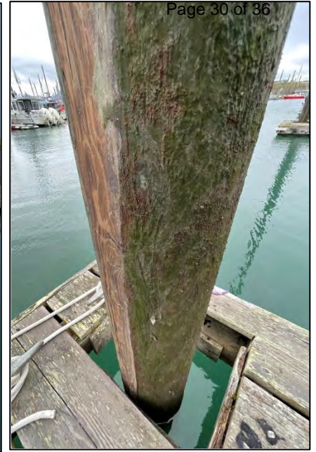
Figure 2.46: Moderate wear on timber piles.
