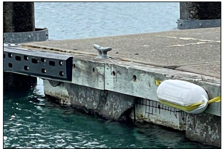
Figure 2.52: Spalled/missing concrete below deck with exposed foam and reinforcing.
