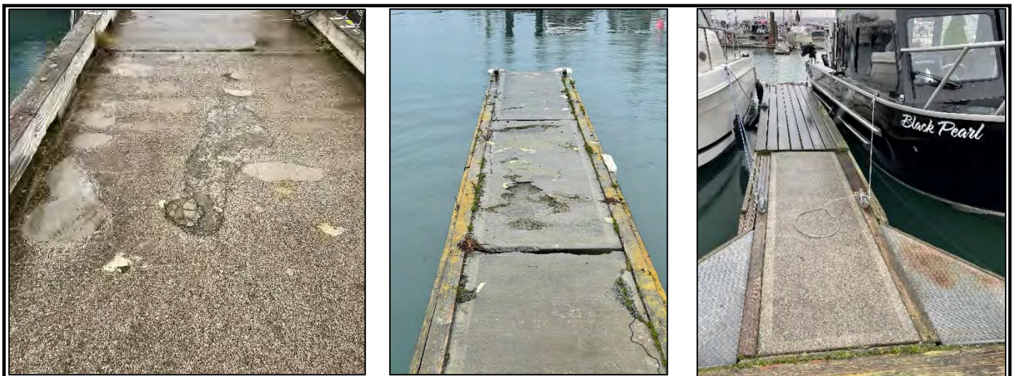
Figure 2.27: Deteriorated concrete surface and concrete repairs, including covering with timber decking.
