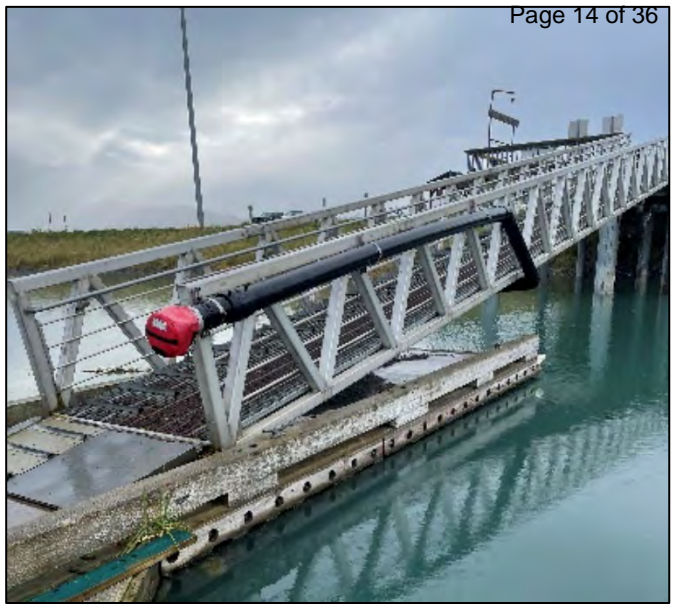
Figure 2.13: Fire system HDPE piping on Ramp 4.
