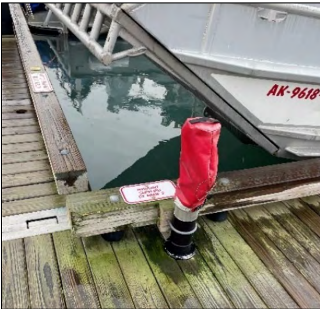
Figure 2.12: Fire suppression system standpipe/hydrant near J Float
