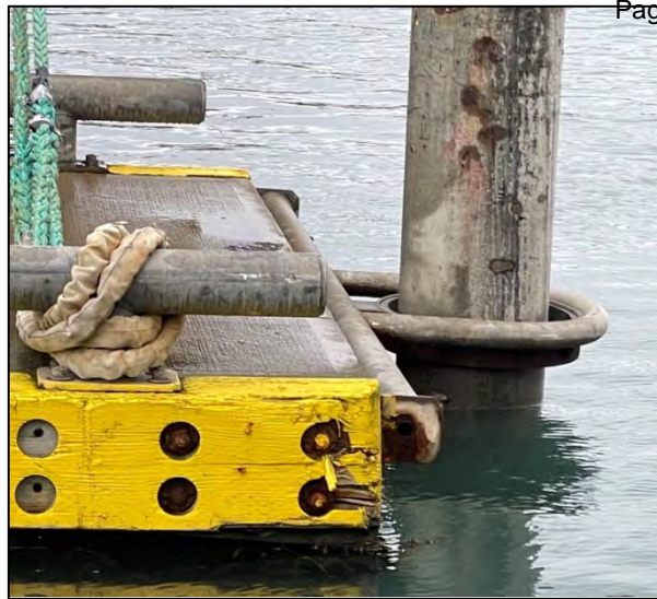
Figure 2.23: Pit corrosion and other areas of active corrosion is evident on some piles
