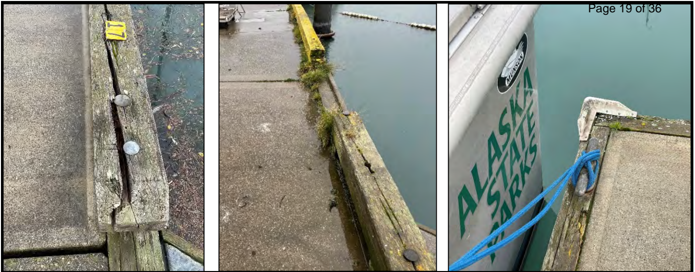
Figure 2.28: Bullrails will major splits and missing section, and cleat mounted in damaged timber waler.
