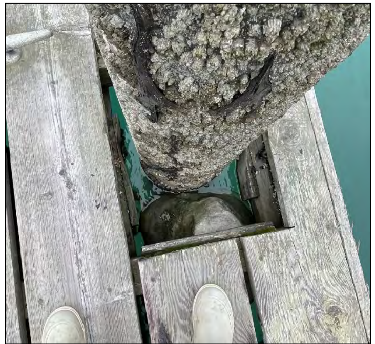
Figure 2.47: View under deck at a pile location. The odd shaped grey item floating between the pile and persons foot is very deteriorated flotation foam that is loose.
