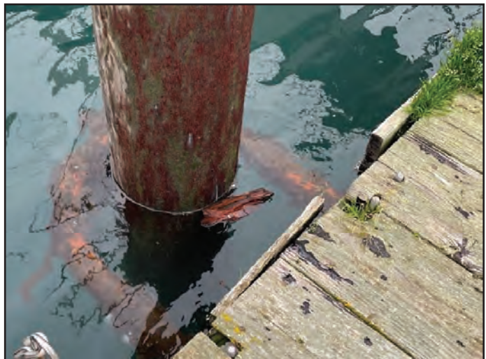
Low freeboard resulting in submerged pile collar. Decking has rot and hardware connections protrude through it.
