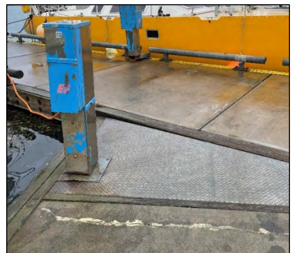
Figure 2.24: Typical power pedestal, many with damaged mounts. Note also typical minor crack in concrete.
