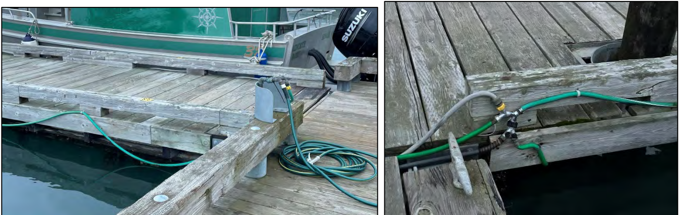
Figure 2.54: Typical water service to main floats provided from headwalk float by various hoses/connections.
