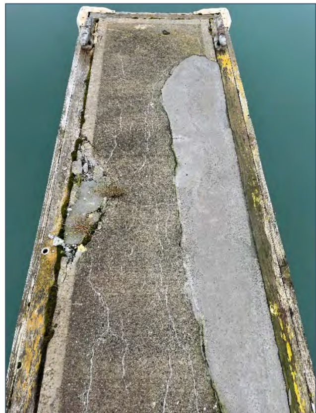
Figure 2.40: Patched concrete and deteriorated water and rubboards on stall floats.
