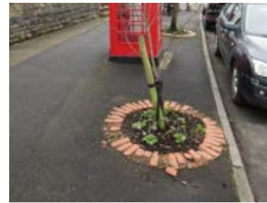
poor brick edging detail on King Street
