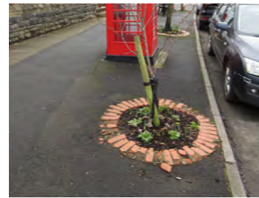
poor brick edging detail on King Street
