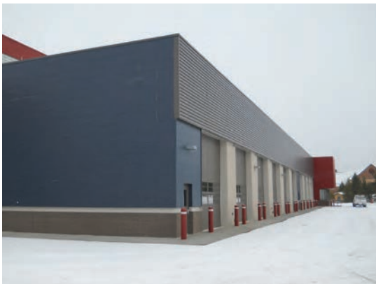
Passive solar wall panel
