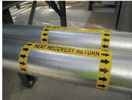
Heat recovery piping
