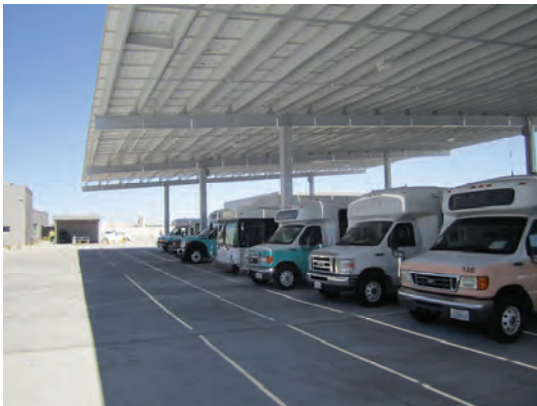
Photovoltaic shade structure
