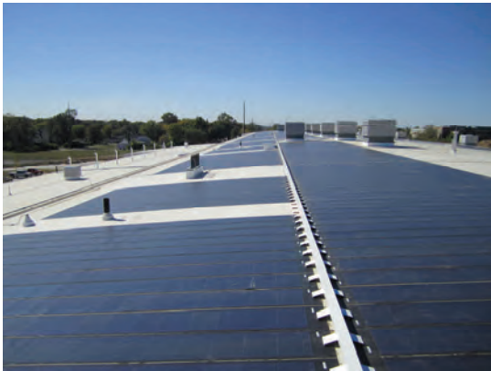
Roof mounted photovoltaic panels
