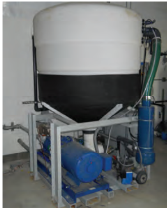
Wash water reclaim system
