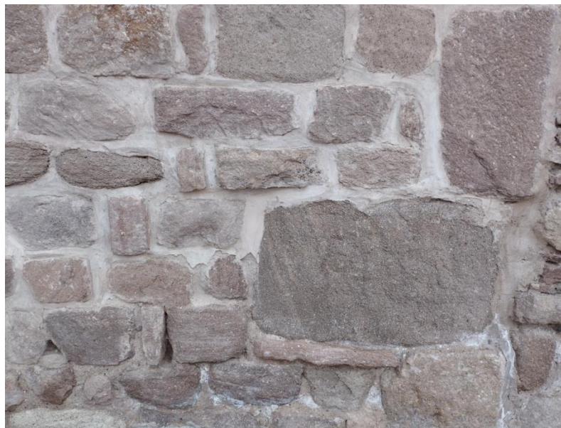
Figure 4. Mortar losses in monument joints
