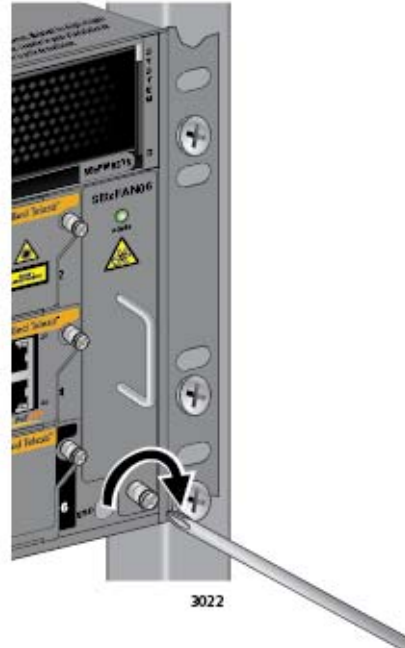
Figure 185. Tightening the Screw on the AT-SBxFAN06 Fan Module
