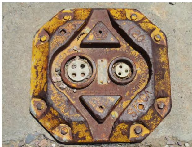
Figure 97. Property 20520, Crouse-Hinds explosion-proof electrical ports in pad, plan view.
