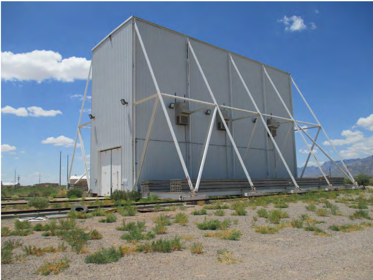
Figure 99. Property 20521 Hera Environmental Shelter, north and east elevations, view to the southwest.
