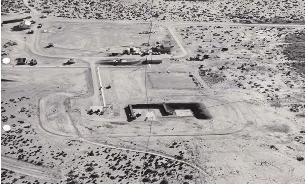
Figure 76. A 1958 aerial photograph of the Hawk area at LC-32 East under construction, Property 20533 at center.
