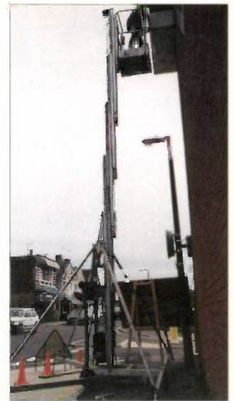
Fig. 3: Even with the outriggers in place the tower takes up little space and can reach up to 12m. The system operates from 115V via an isolating transformer which is hired along with the platform (see text).
