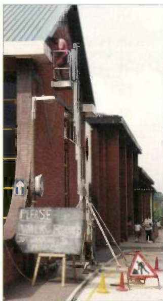
Fig. 1: No...he's not 'jet washing' but using a portable electric drill! This portable American-made telescoping mini-tower could prove useful in antenna maintenance and helps improve safety (see text).
