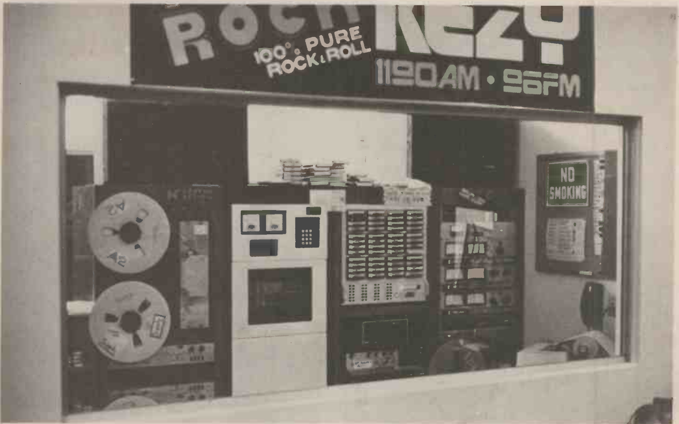
Inside this air conditioned room is the equipment used for the automated FM broadcasts. The tape deck on the upper left contains all of the verbal 'breaks' between records. The lower deck has all of the music. The cartridge bank in the centre holds all of the pre-recorded adverts. Below that the micro-processor unit that controls everything.
