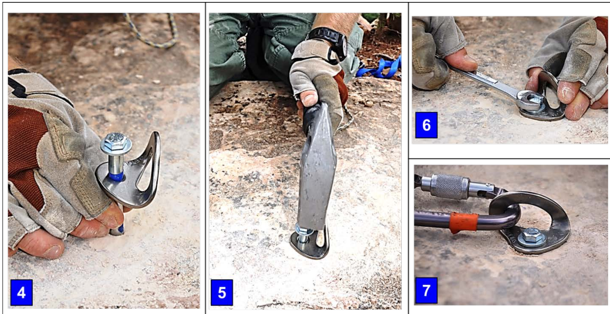
Figure 132- Bolting Techniques (cont'd); 4.) Insert the bolt and hanger 5.) Tap the bolt into the drilled hole until it is firmly seated with the hanger against the rock surface. 6.) Tighten with appropriate amount of torque 7.) Test the placement for strength.
