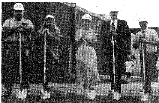
Ready to start digging for the new Bristol Grade School addition are school board members Jack Spencer, member; Jeanie Lindstrom, clerk; Barb Boldt, vice president; Rich Bizak, president; and Ed Becker, treasurer. (Scott Koker photo)
