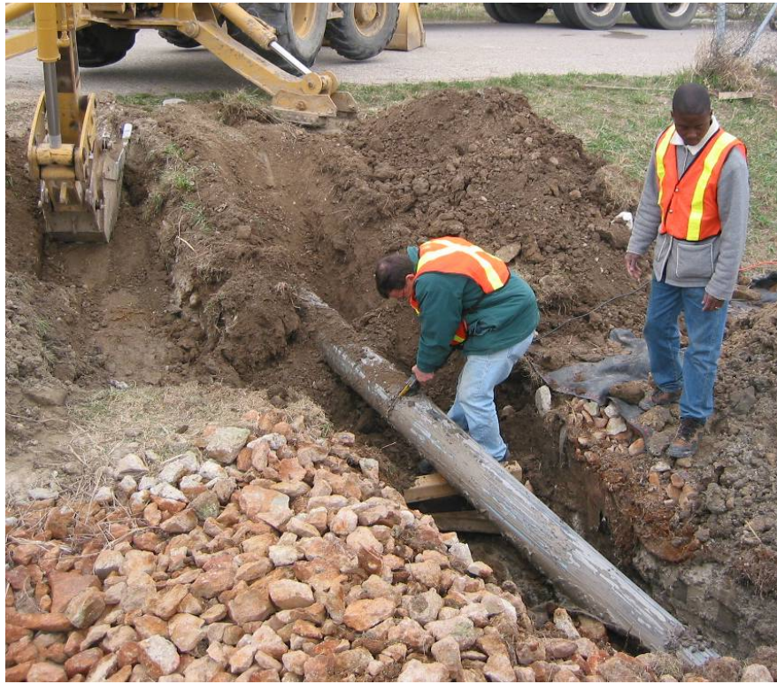
Figure 5.38: Backhoe inadvertently caused additional pipe deflection on CO test section
