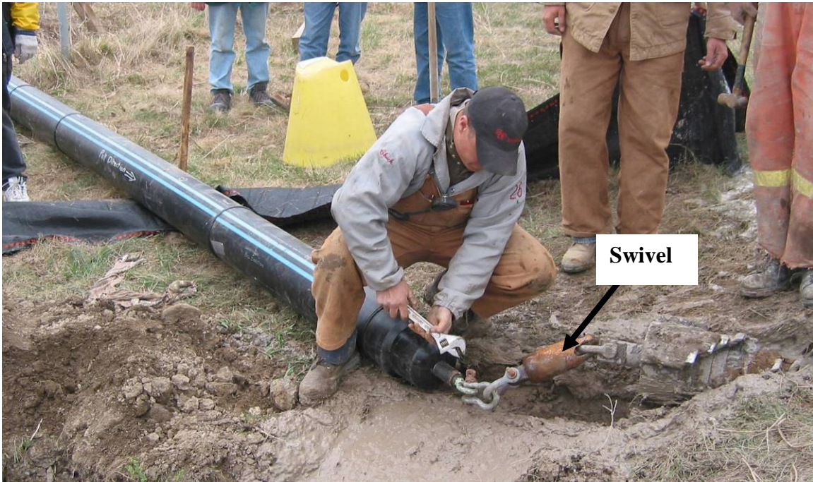
Figure 5.8: HDD installed HDPE pipe ready to be pulled through the pre-reamed bore
