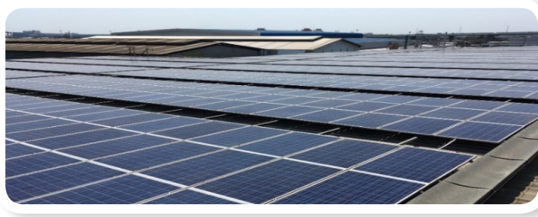
Project Site: Saha Thai Steel Pipe Public Co., Ltd. (SHT), Samut Prakarn Province, invested by UACE
