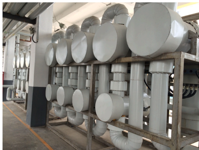
Fig. 15. 10 kt/a acetonitrile separation plant with the integration of distillation and molecular sieve membrane in Shandong Huihai Company.
