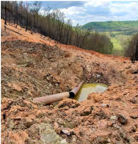
Figure 1. Ruptured pipeline. (Source: BGC Engineering USA, Inc.)
