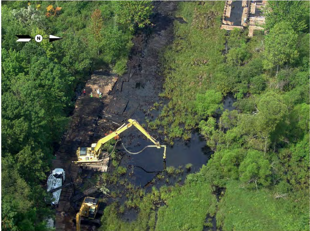
Figure 4. Cleanup efforts in an oil-soaked wetland near the rupture site. Saturated soil complicated the cleanup and excavation efforts. An excavator with a vacuum attachment is shown situated on wooden matting near the rupture site.
