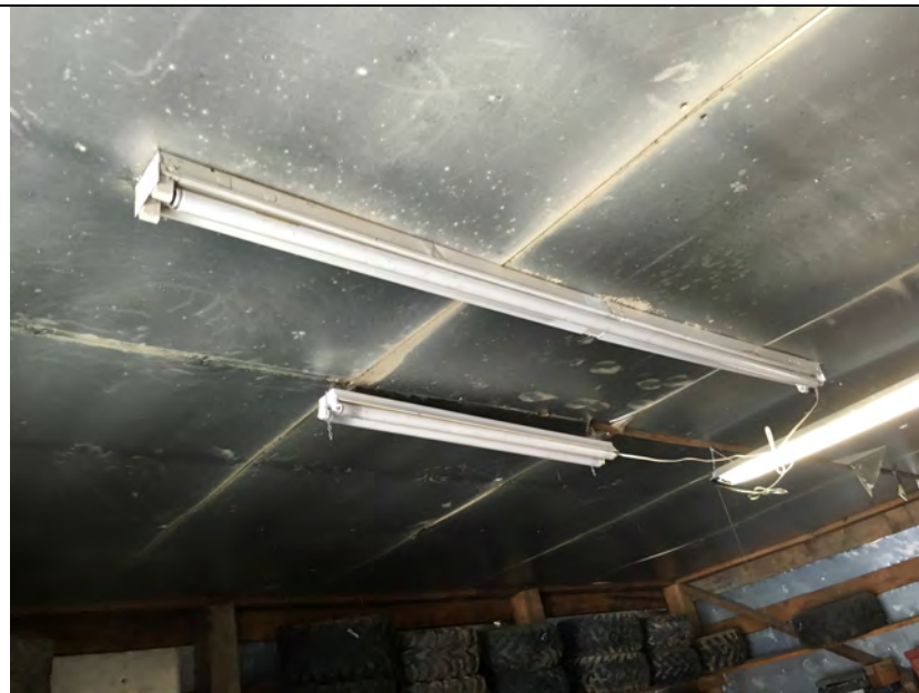
8 ft fluorescent light fixture.
