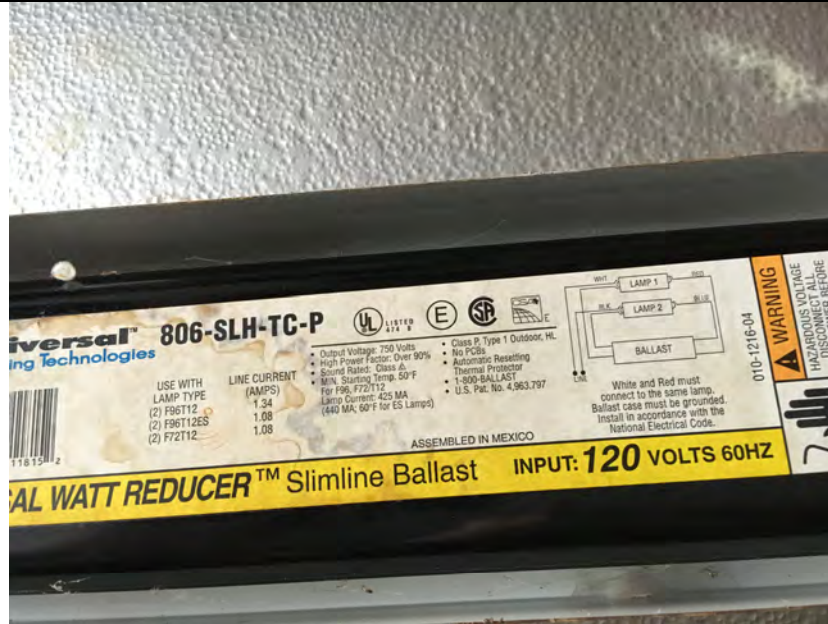
Light ballast labeled "No PCBs" in 8 ft fluorescent light fixture.
