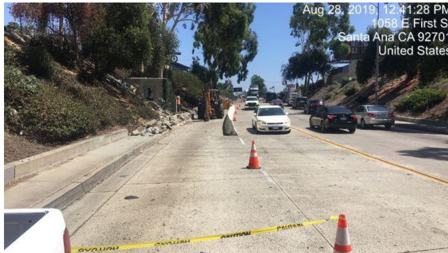
First Street Lift Station
