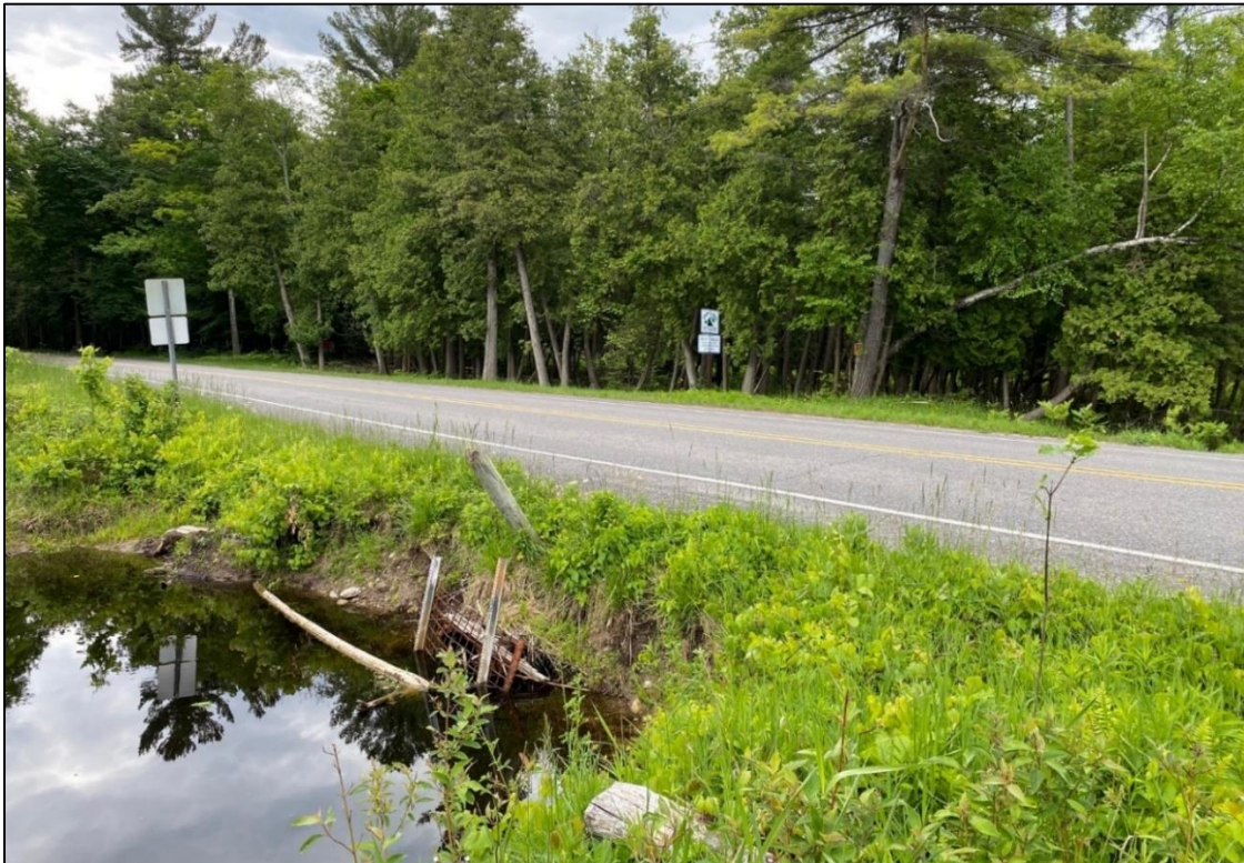
Figure 8. Crossing #4 (Tucker Lake Outlet), downstream section, looking south-southeast with CR 675 in foreground.
