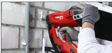
Conduits and light-duty pipes
