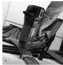
Conduits & pipes with metal or textile band
