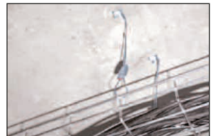
Light weight Cable Trays / Lights
