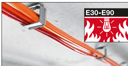
Circuit integrity system (CIS) application with fire rating and load data according to AbP
