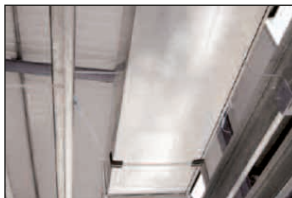
Square Air Ducts
