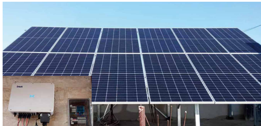
30kW Solar System in Israel (XG30KTR)
