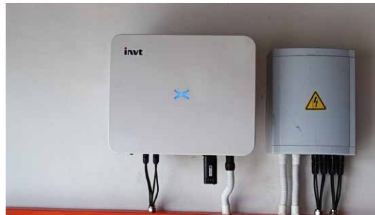
25kW Solar System in Malaysia (XG25KTR)
