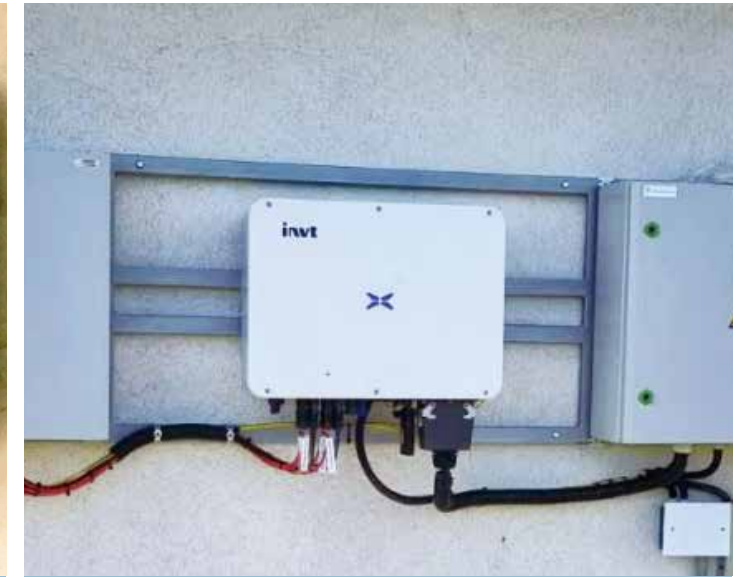
30kW Solar System in Serbia (XG30KTR)
