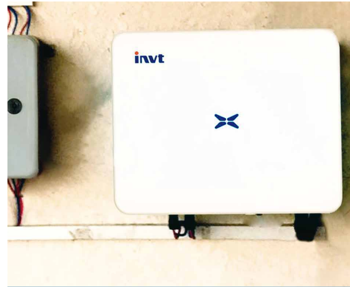
10kW Solar System in Armenia (XG10KTR)
