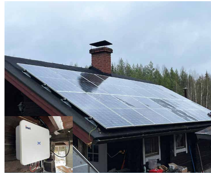
8kW Solar System in Finland (XG8KTR)
