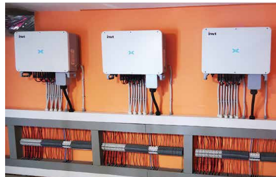
180kW Rooftop PV Plant in Lebanon (XG60KTR)
