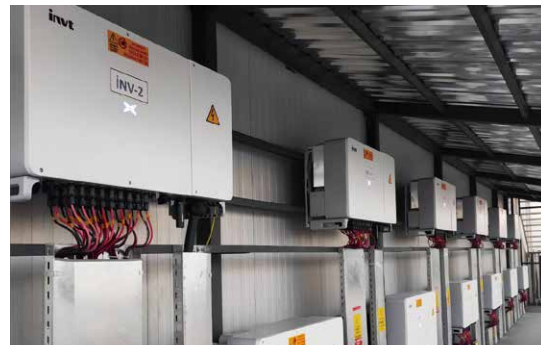
2MW Rooftop PV Plant in Türkiye (XG110KTR)
