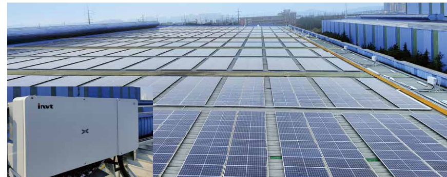
13.86MW Rooftop PV Plant in Hubei, China (XG136KTR-X)
