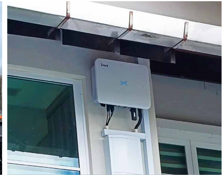
12kW Solar System in Malaysia (XG12KTR)
