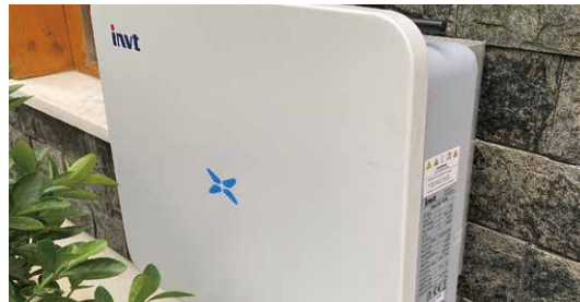
10kW Solar System in Romania (XG10KTR)
