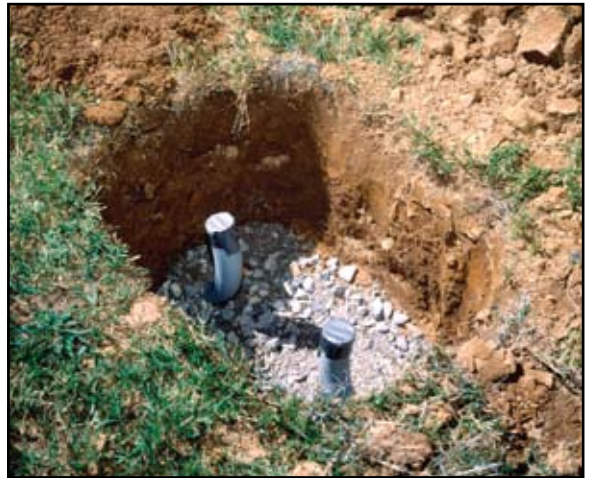
Excavate 6 inches deeper than the depth of the enclosure and add 6 to 8 inches of gravel or crushed rock (1.02).
