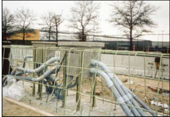
QUAZITE® enclosures are embedded in concrete highway median barriers.
