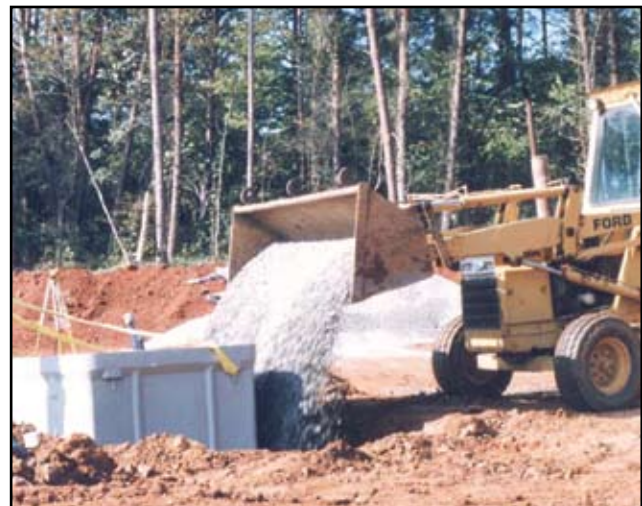
Place gravel in the enclosure and around the side. Lift enclosure to let gravel run underneath (4.04, 4.05).
