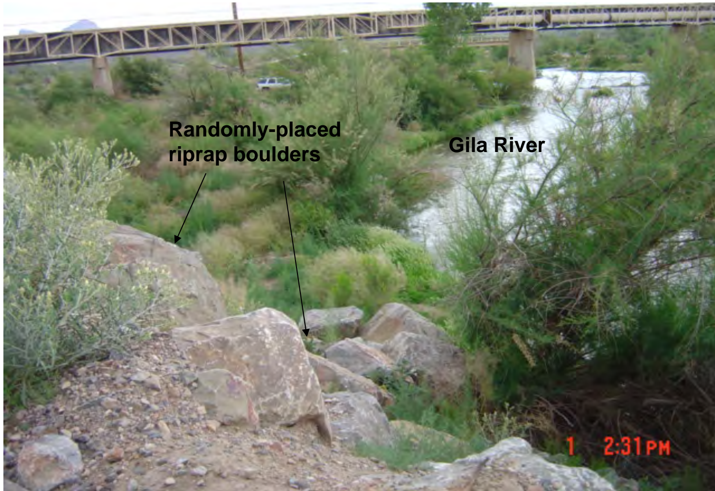
View near southwest corner of North Emergency Tailings Pond and Gila River. Railway trestle in background. Randomly placed riprap boulders in foreground along pond berm.
