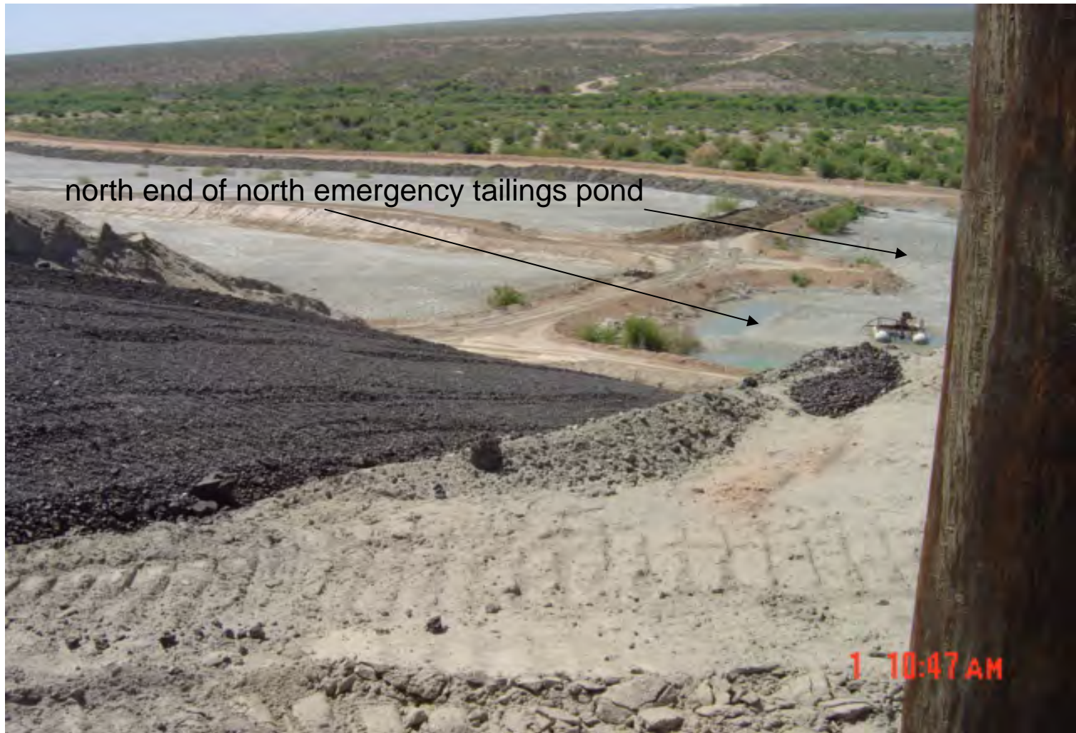
Erosion repairs to lower slope near southwest corner of Impoundment AB/BC using crushed furnace slag.
