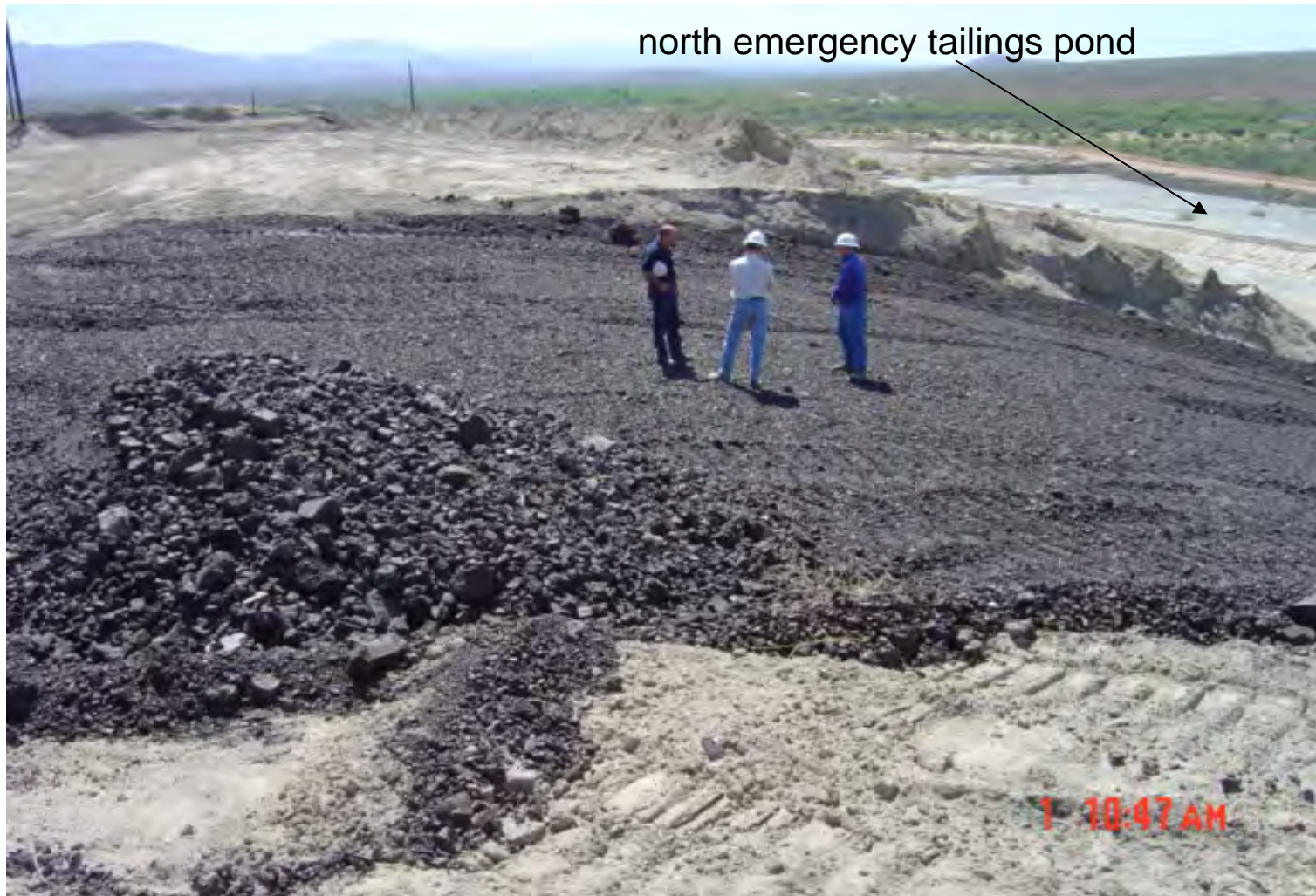
Erosion repairs to lower slope near southwest corner of Impoundment AB/BC using crushed furnace slag.
