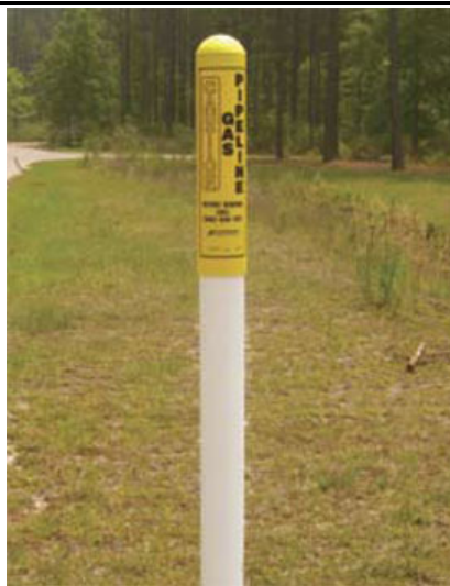
Figure 3.30 Example of a marker indicating pipeline below ground
